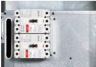
Additional subfeed with aux and shunt trip
