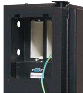
400 and 500 kVA comm port access
