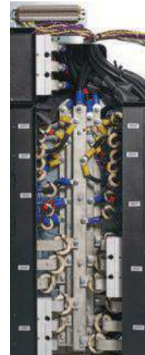
400 and 500 kVA Main Bus (patent pending)
